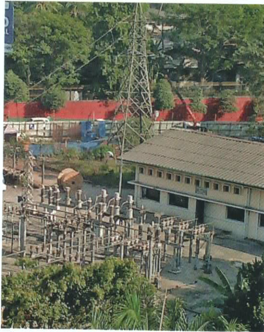
Efforts are under way to develop and modernise the electrical grid
