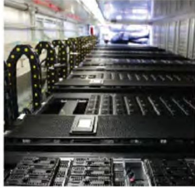
Animal Logic – Sydney, AU Bringing characters to life for the silver screen with prefab data center solutions
